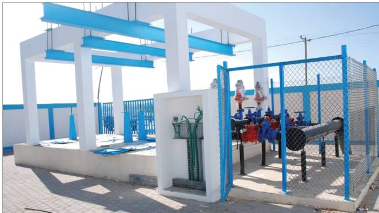
39- Al Mughraqa sewage pumping station- Gaza
